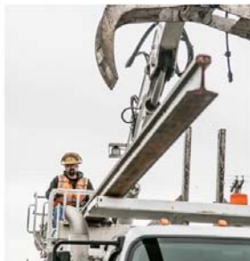
Automated Rail Unloading
