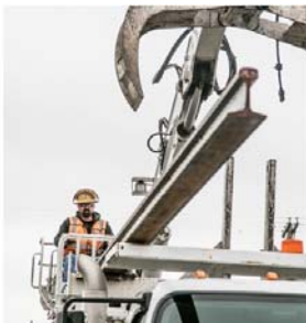
Automated Rail Unloading
