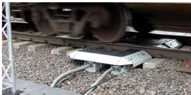
Wheel profile detectors capture critical information every time a train passes by.
