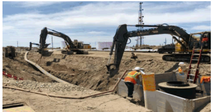
Crews work on a new industrial wastewater system in JR Davis Yard.
